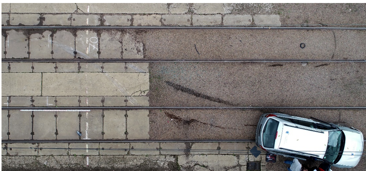
Obr. 16 - Stopy na povrchu trati. Fig. 16 – Traces on the track surface.
