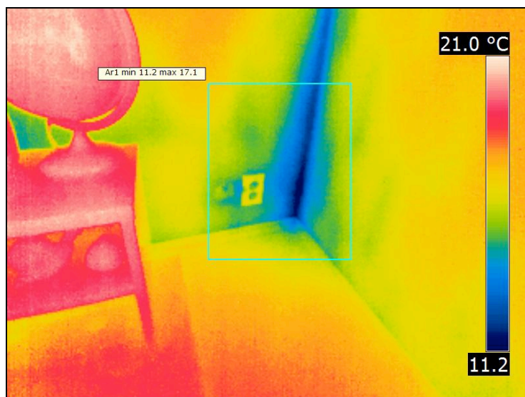
Obr. 2 – Termogram s nízkou povrchovou teplotou Fig. 2 – The thermogram of the low surface temperature
